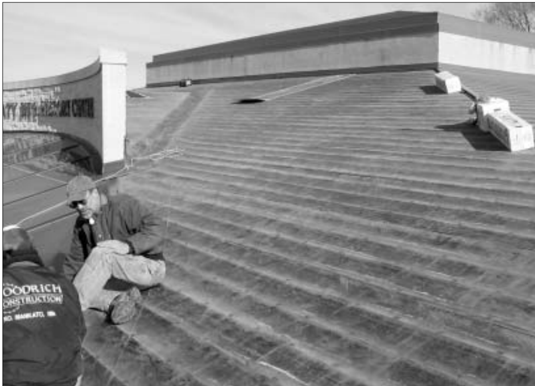
Ron Goodrich (right) and Randy Dinsmore of Goodrich Construction during the reconstruction of the roof at the TSHC. Thanks to their good work we are "weatherproof" for the winter.
